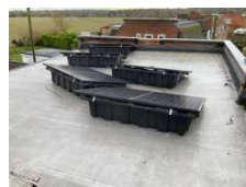
Flat roof space where solar panels were located and had moved during the high winds
